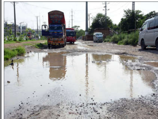
ISLAMABAD: Motorists facing difficulties due to damage service road along Karnal Sher Khan Shaheed Road after the heavy monsoon rain in the Federal Capital.
