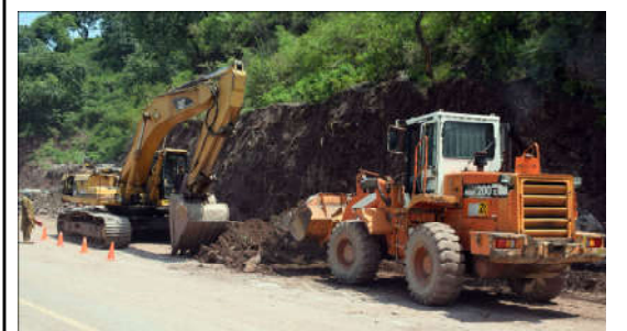
MUZAFFRABAD: Labourers are busy in construction work with the help of heavy machinery alongside a road in the city.
