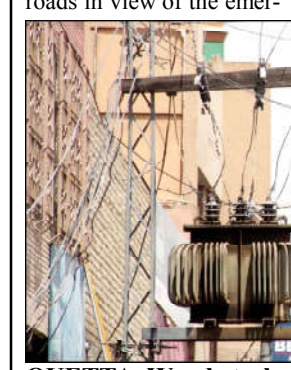
QUETTA: Wapda technician is installing electric wires on an electric pole after damages, at Sarki road in Quetta.
