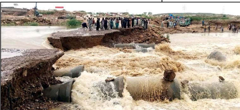
HUB: View of destruction at Hub River Causeway road once again due to floods causing of poor sewerage system creating problems for commuters and residents, after heavy rainwater flowed in area due to heavy downpour of monsoon season, showing negligence of concerned authorities, in Hub.
