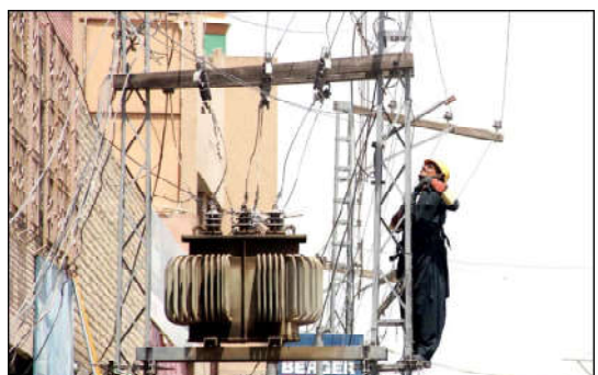
QUETTA: Wapda technician is installing electric wires on an electric pole after damages, at Sarki road in Quetta.
