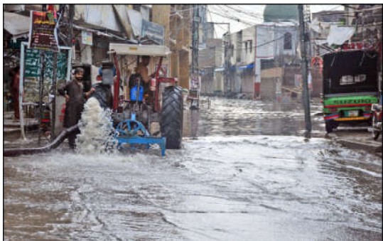
RAWALPINDI: Workers are busy in draining accumulated rain water after heavy rain at Imam Bara road area, in morning hours in the city.
