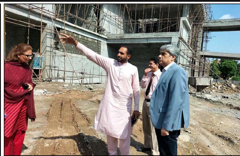
ISLAMABAD: Federal Secretary Health Nadeem Mahbub visited the under construction emergency unit in PIMS.
