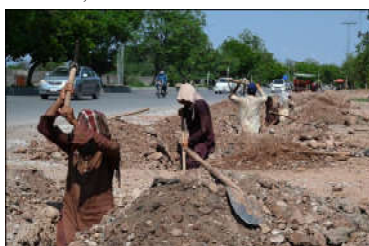
ISLAMABAD: Laborers busy digging at roadside for installing new pipeline at Lehrar Road.
