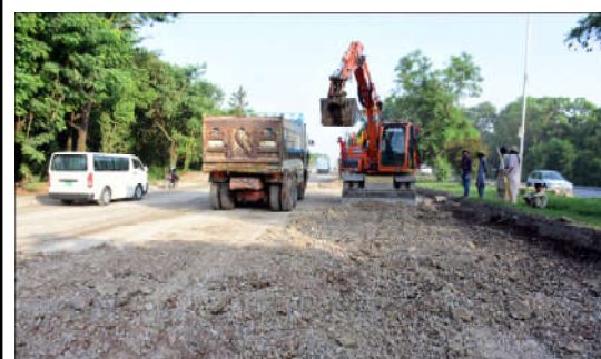
ISLAMABAD: Work in progress on Park Road expansion project in the Federal Capital.
