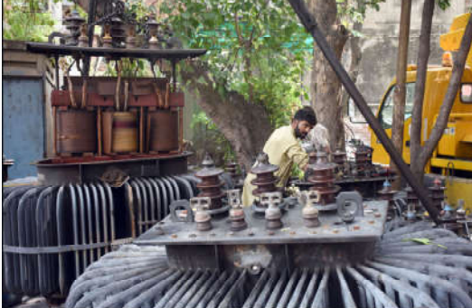
LAHORE: AWPDA engineer is busy in repairing Transformers at G.R.O in the Federal Capital.
