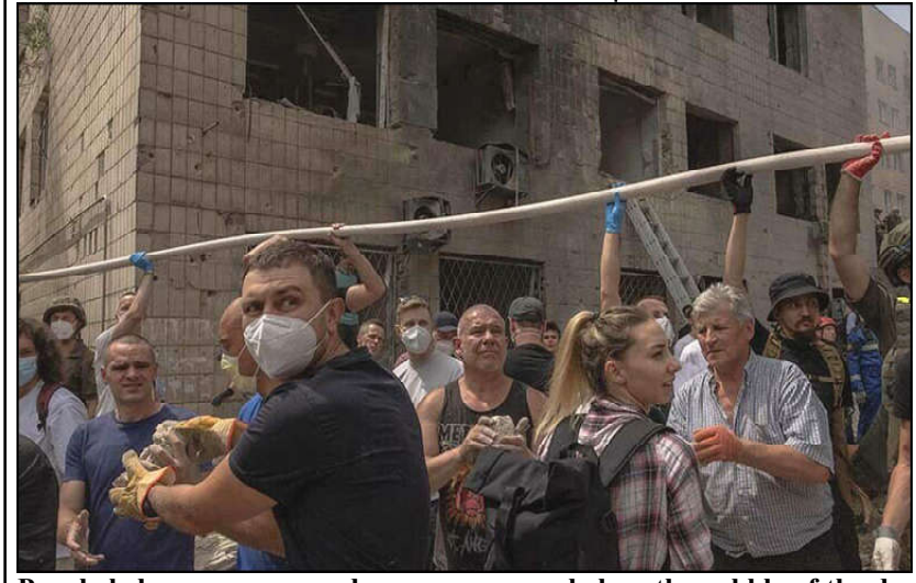
People help emergency and rescue personnel clear the rubble of the destroyed building of Ohmadyt Children's Hospital following a Russian missile attack in the Ukrainian capital of Kyiv.
