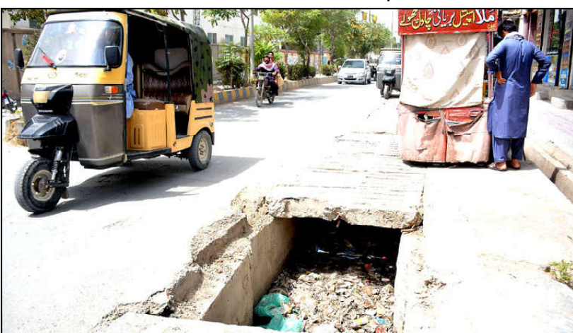
QUETTA: A view of the cover of the manhole is missing in front of the Civil Hospital which may cause any accident that need the attention of concerned authorities
