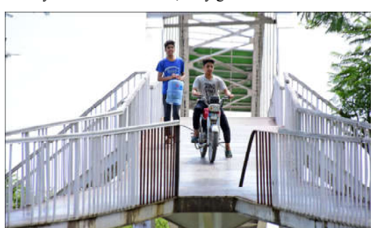
ISLAMABAD: A young boy riding motorcycle on a broken foot pedestrian bridge alongside 7th Avenue, in the Federal Capital, which may cause any incident any times as needs to attention for concern authority.
