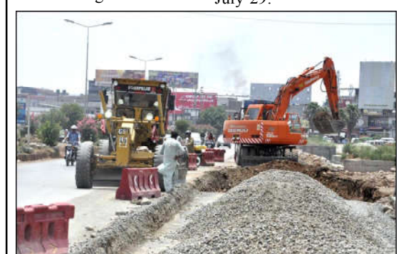
ISLAMABAD: Heavy machinery being utilized for expansion work of Club Road during development work in Federal Capital.
