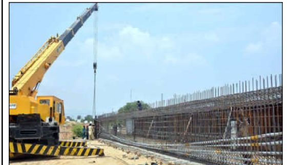
ISLAMABAD: Labourers busy in construction work of flyover at under construction 10th Avenue during development work in Federal Capital.
