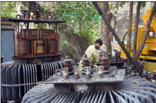
LAHORE: AWPDA engineer is busy in repairing Transformers at G.R.O in the Federal Capital.
