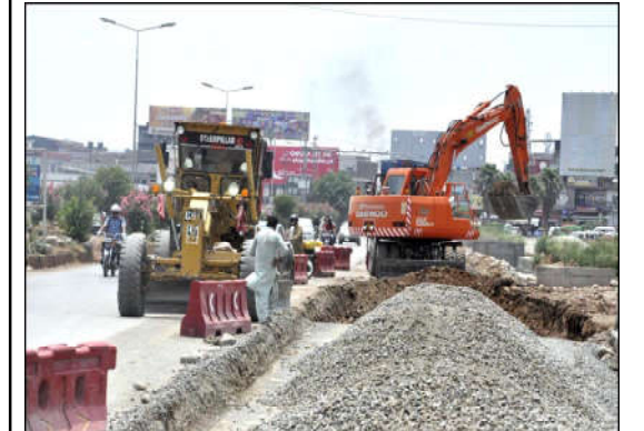
ISLAMABAD: Heavy machinery being utilized for expansion work of Club Road during development work in Federal Capital.
