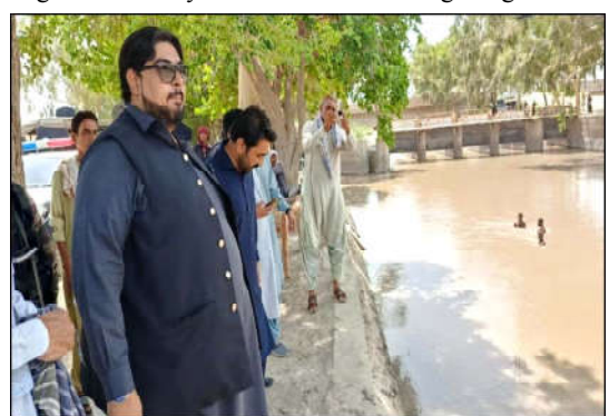
USTA MUHAMMAD: Director General PDMA Jahanzeb Khan and Assistant Commissioner inspecting Kerthar canal
