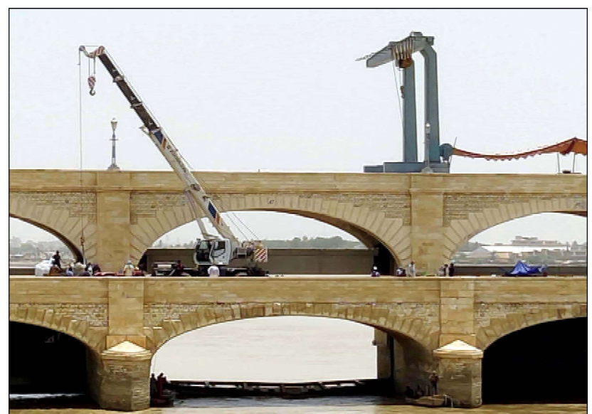
SUKKUR: Repair work of Sukkur Barrage Gate No. 47 and 44 is in progress, these gates have been severely damaged by water flow, in Sukkur
