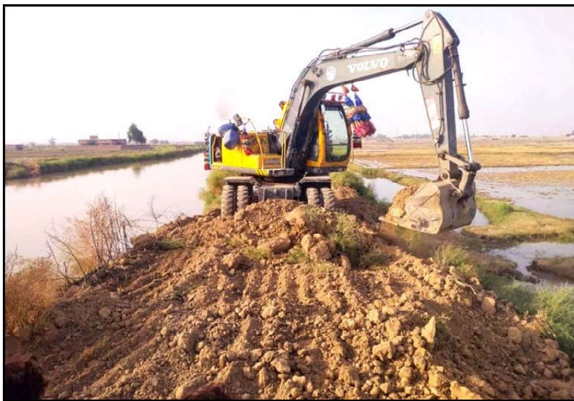
On the directives of Executive Engineer Drainage Naserabad Zone Mudassar Zafar Khosa crack of temple drainage being filled
