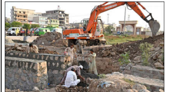
ISLAMABAD: Labourers busy in construction work at Park Road with the help of heavy machinery during development work in the Federal Capital.
