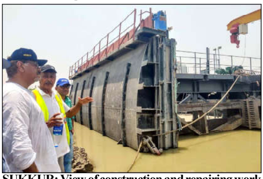
SUKKUR: View of construction and repairing work of damage to gates No 44 and 47 of Sukkur Barrage while the Kisan Gate (temporary gate) to the barrage for replace damaged gates of Sukkur Barrage in Indus River, in Sukkur.
