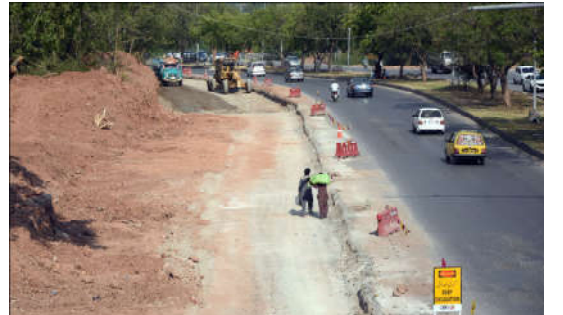
ISLAMABAD: Labourers are busy in construction work of Chak Shahzad road during development work in the Federal Capital.
