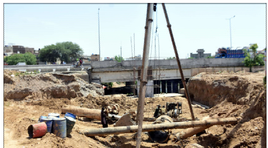
ISLAMABAD: Construction work on a project on Karnal Sher Khan Road is in progress in the Federal Capital, a 5-kilometre road is being constructed from Katarian Bridge on L.J.P Road to Srinagar Highway near the intersection of G-9 and G-10.
