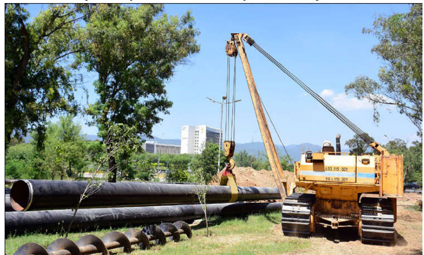
ISLAMABAD: Labourers are busy installing new gas pipeline with the help of heavy machinery at Zero point area during development work.
