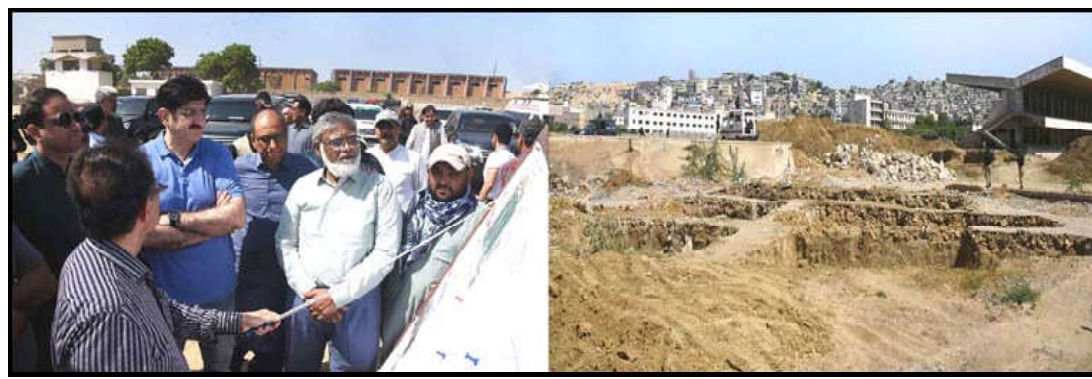
KARACHI: Sindh Chief Minister, Syed Murad Ali Shah being briefed about the progress of under construction Bakhtiari Sports Complex at District Central during his inspection visit, in Karachi.
