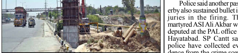
ISLAMABAD: Labourers busy in construction work of flyover at under construction 10th Avenue during development work in Federal Capital.
