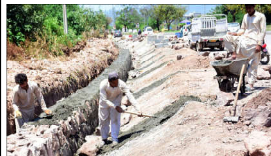
ISLAMABAD: Labourers working on sewage water project on Chak Shahzad road in the Federal Capital.
