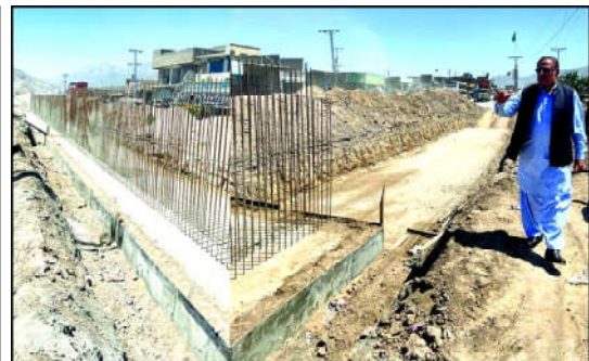
QUETTA: Provincial Minister for C&W Mir Saleem Ahmed Khosa reviews under construction work of Custom and Gahi Khan Flyover.
