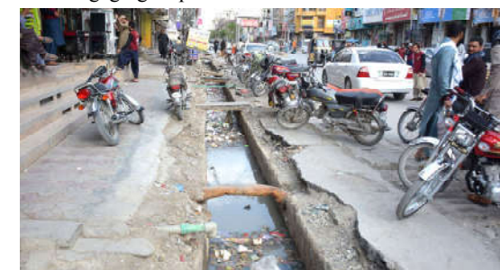
QUETTA: A view of the open sewerage nullah in front of shop may cause any mishap that need the attention of concerned authorities.
