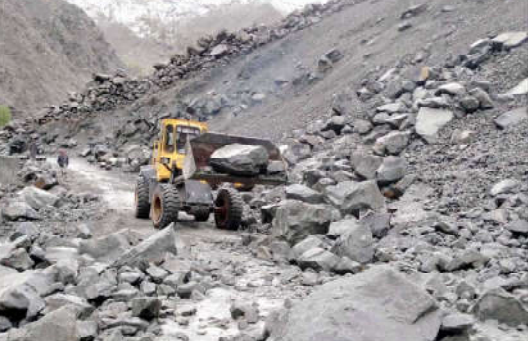
GILGIT: Workers of Gilgit-Baltistan Disaster Management Authority and GBPWD busy in clearing blocked road of Astore after heavy rain and land sliding in the area.
