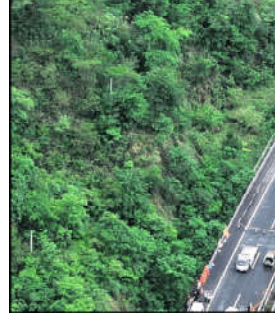
Part of an expressway collapsed in south China's Guangdong Province on after heavy rains.
