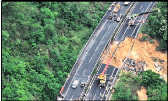
Part of an expressway collapsed in south China's Guangdong Province on after heavy rains.
