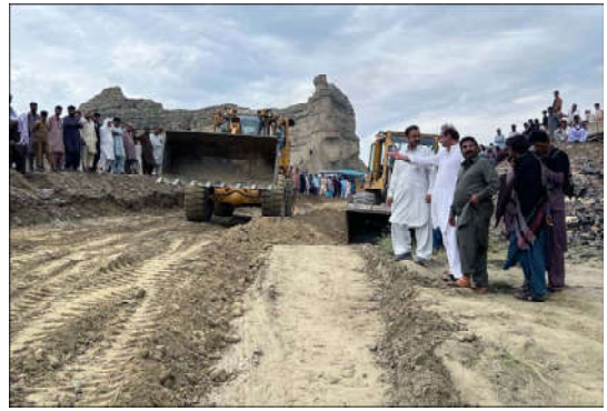
HUB: Heavy machineries and laborers busy in construction work of Causeway crossing road completely destroyed after flood in Hub River during recent heavy downpour of monsoon, under supervision NHA, located on Gwadar Coastal Highway.
