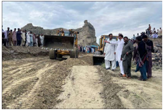
HUB: Heavy machineries and laborers busy in construction work of Causeway crossing road completely destroyed after flood in Hub River during recent heavy downpour of monsoon, under supervision NHA, located on Gwadar Coastal Highway.
