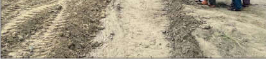
HUB: Heavy machinery and laborers busy in construction work of Causeway crossing road completely destroyed after flood in Hub River during recent heavy downpour of monsoon, under supervision NHA, located on Gwadar Coastal Highway.
