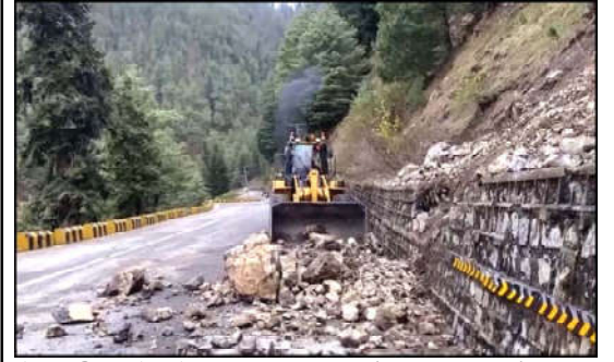
ABBOTTABAD: Heavy machinery removing debris after land sliding due to heavy downpour, located on Nathiagali road in Abbottabad.
