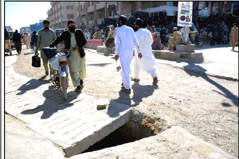
QUETTA: Commuters pass through nearby an open sewerage main hole that may cause any accident specially in night hours, showing the negligence of concerned departments, at Bacha Khan Chowk in Quetta.
