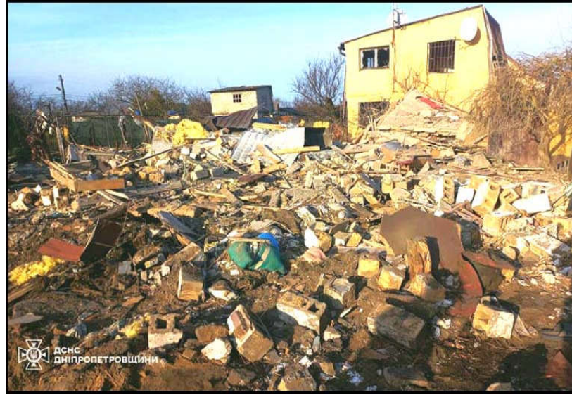
A view of residential buildings damaged during a Russian missile strike in Kamianske, a city in Ukraine's Dnipropetrovsk region.
