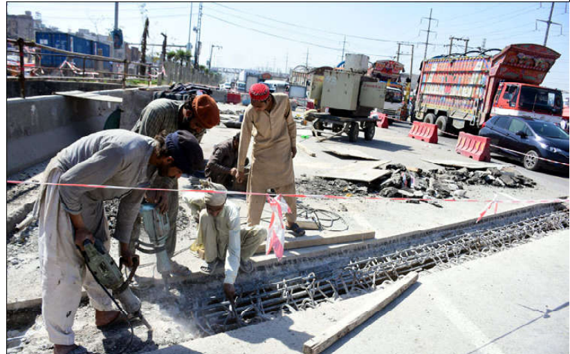
ISLAMABAD: Labourers are working on maintenance of a bridge on Colonel Sher Khan Shaheed Road near Pirwadhai stop, one side of the bridge was collapsed owing to the heavy traffic.
