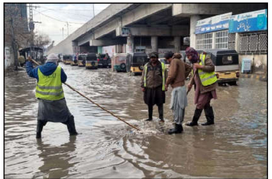
QUETTA: Workers of Quetta Metropolitan Corporation (QMC) are busy in cleaning and draining the stagnant rainwater after heavy downpour of winter season.
