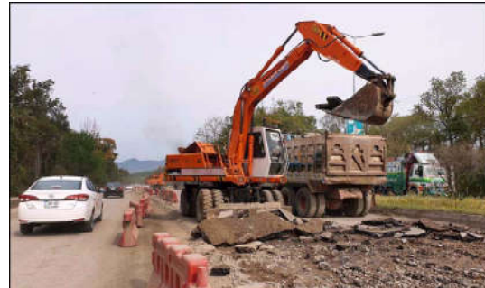
ISLAMABAD: Heavy machinery being used to expand a road at Chak Shahzad in the Federal Capital.
