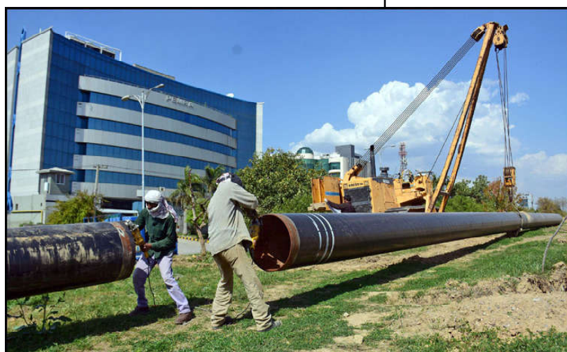
ISLAMABAD: Labourers working on new gas pipeline project along Sector G-8 in the Federal Capital.
