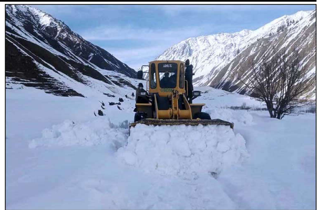
GILGIT: Heavy machinery being used to remove snow from the blocked road of Mir Malik area Astore Valley.
