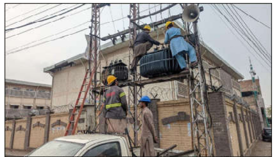
PESHAWAR: PESCO workers are busy repairing the transformer in the Tehsil area.
