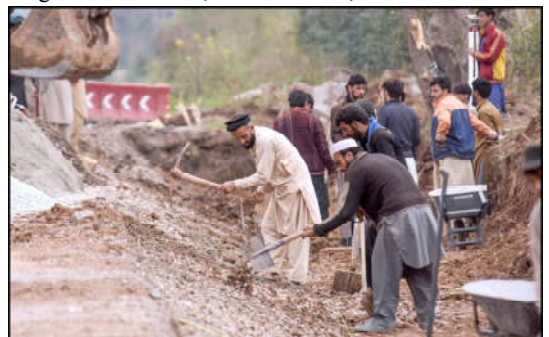
ISLAMABAD: Labourers working on expansion of Chak Shahzad Road in the Federal Capital.
