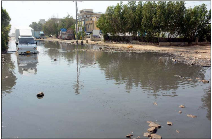
KARACHI: Inundated road by overflowing sewerage water, creating problems for residents and commuters, showing negligence of concerned authorities, located on Korangi S.M Munir road in Karachi.
