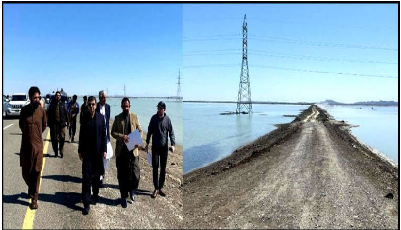
GWADAR: Chief Secretary Balochistan Shakeel Qadir Khan inspecting roads damaged due to recent rains
