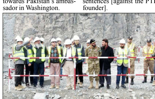
Chairman WAPDA Lt. Gen (Retd) Sajjad Ghani inspecting ongoing construction work during his visit to Diamer Basha Dam.
