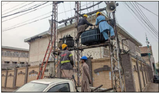
PESHAWAR: PESCO workers are busy repairing the transformer in the Tehsil area.
