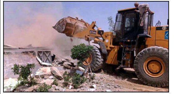
KARACHI: Anti encroachment operation in progress removed illegal encroachment during anti encroachment drive under the supervision of Karachi Development Authority (KDA), at Surjani Town Sector 13/7 in Karachi.
