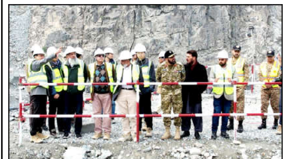
Chairman WAPDA Lt. Gen (Retd) Sajjad Ghani inspecting ongoing construction work during his visit to Diamer Basha Dam
