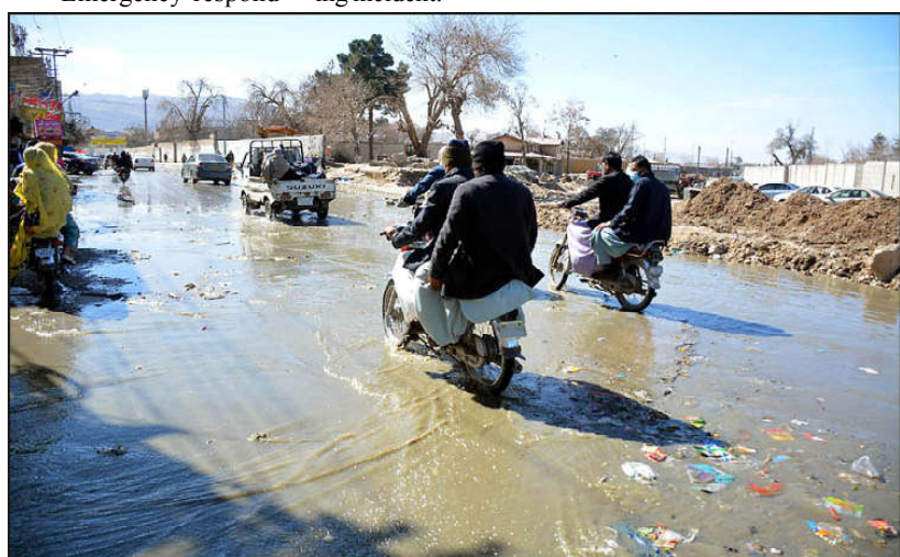
QUETTA: Vehicles passing through sewerage water accumulated on the Jinnah road need the attention of concern authorities.
