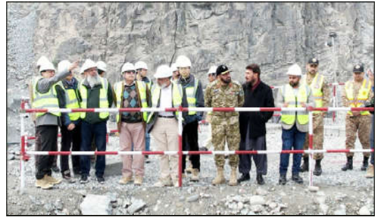
Chairman WAPDA Lt. Gen (Retd) Sajjad Ghani inspecting ongoing construction work during his visit to Diamer Basha Dam.
