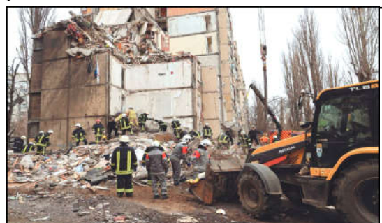
Rescuers work at the site of a heavily damaged apartment building in Odesa, following a Russian drone attack.
